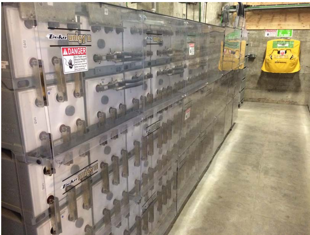
Figure 13. The National Park Service budgets, ideally, $100,000 per year for O&M of this PV energy storage system (308 kW PV; 1,920 kWh battery) on Alcatraz Island. Photo by Andy Walker, NREL
