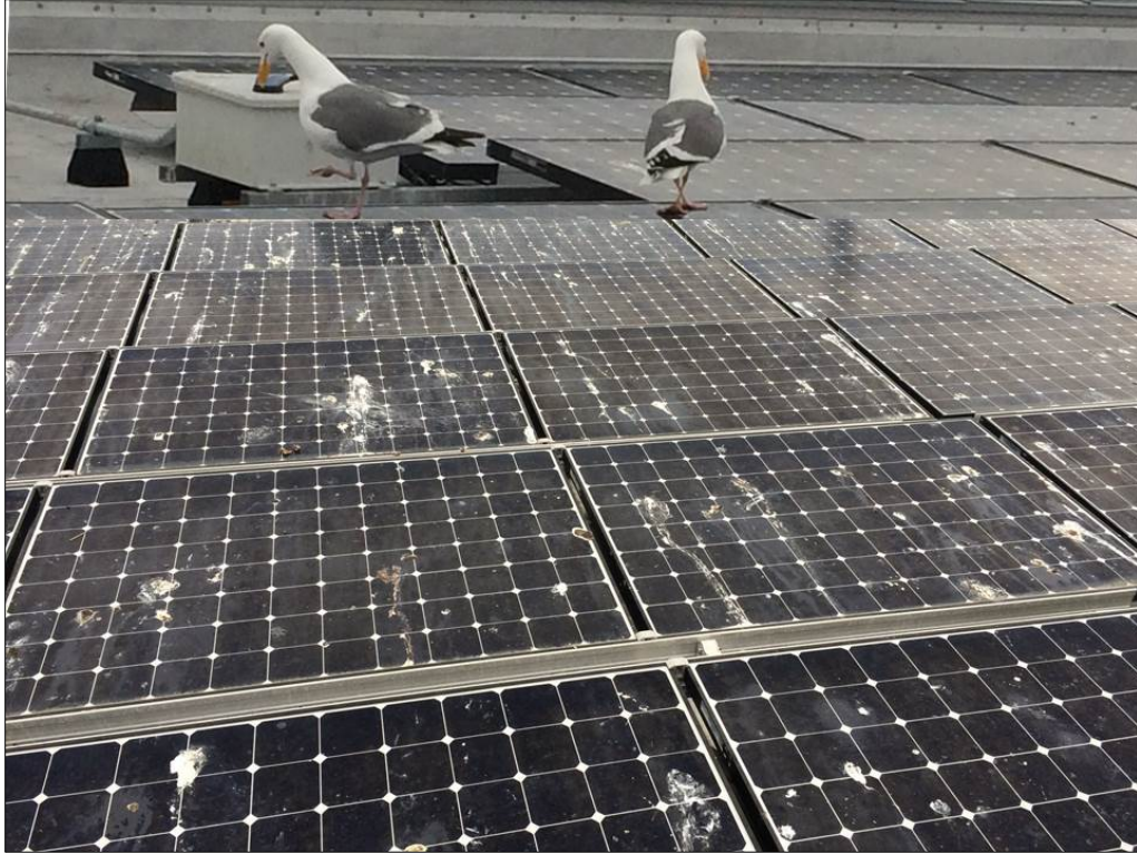
Figure 8. Bird populations are a source of soiling, as well as nests that need to be removed and seeds that can sprout on arrays. Photo by Andy Walker, NREL
