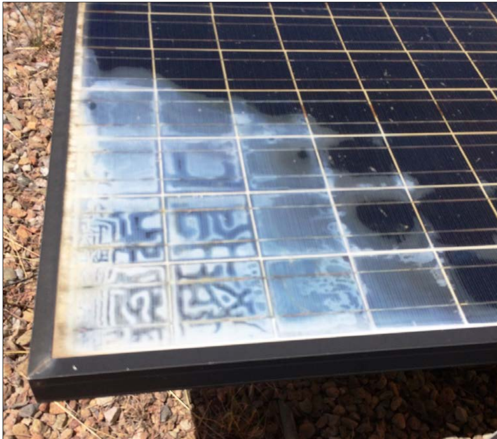
Figure 14. Failure in materials and workmanship, such as encapsulant of this module, are often covered by product manufacturer's warranty. Photo by Andy Walker, NREL
