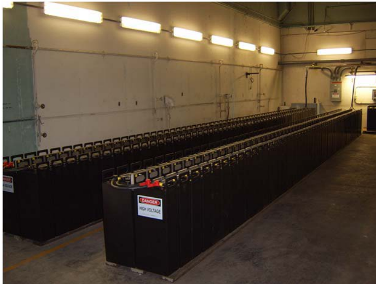
Figure 1. Two strings of batteries are recommended in design to allow O&M service of one string while the other string serves the purpose. Photo by Andy Walker, NREL
