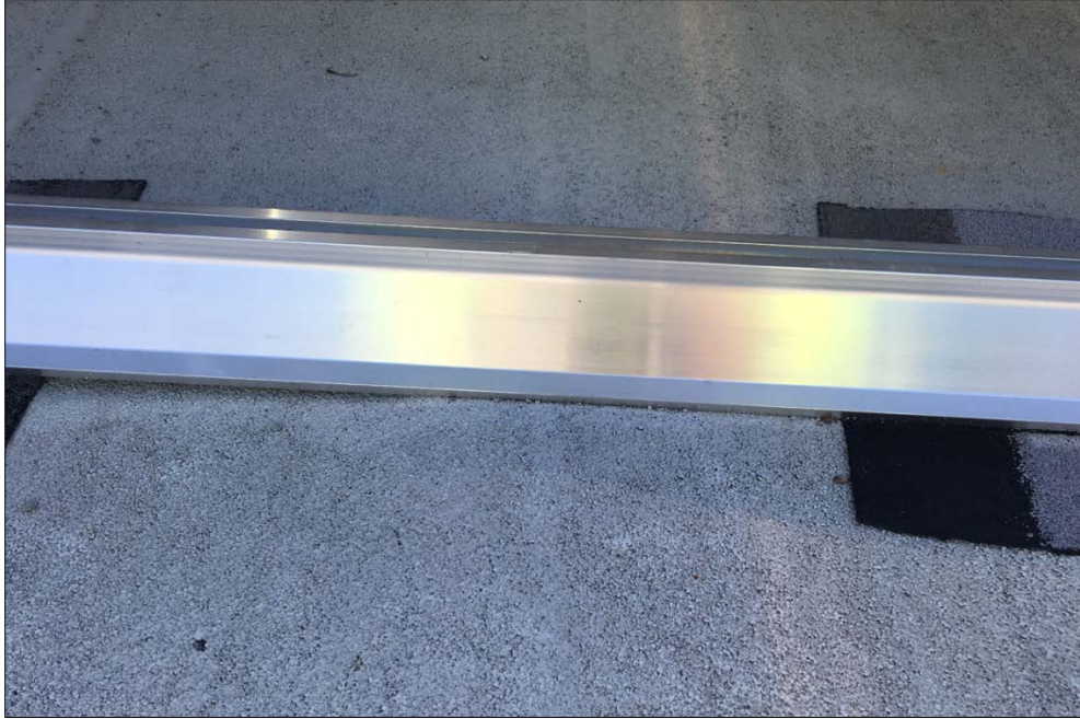
Figure 3. A best practice is to run a slip sheet continuously under rack members to avoid direct contact with the roof membrane. In this photo, direct contact of the rack is cutting into the roof surface. Photo by Norm Crouse, Lightbox Energy
